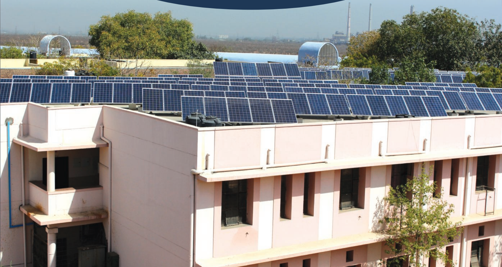
Grid Connected Rooftop Solar PV Power Plant at Department of Renewable Energy, RTU Kota.
